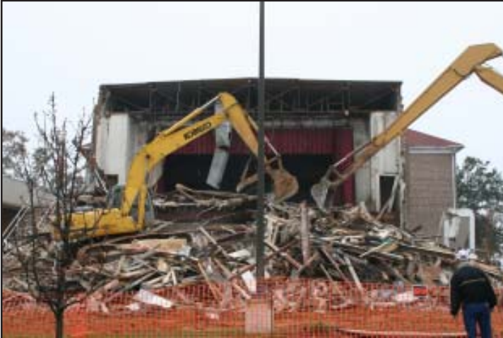
Track-hoes work to demolish historic Moody Hall auditorium. Demolition took place during the Christmas break.
