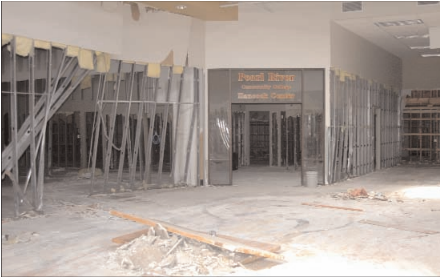
WAVELAND - Cleanup operations have been underway for some time at the Hancock Center, which was devastated by Hurricane Katrina. Plans are to have portable classrooms operational in the Center parking lot for the 2006 spring semester. Photo by Pamela Luke.
