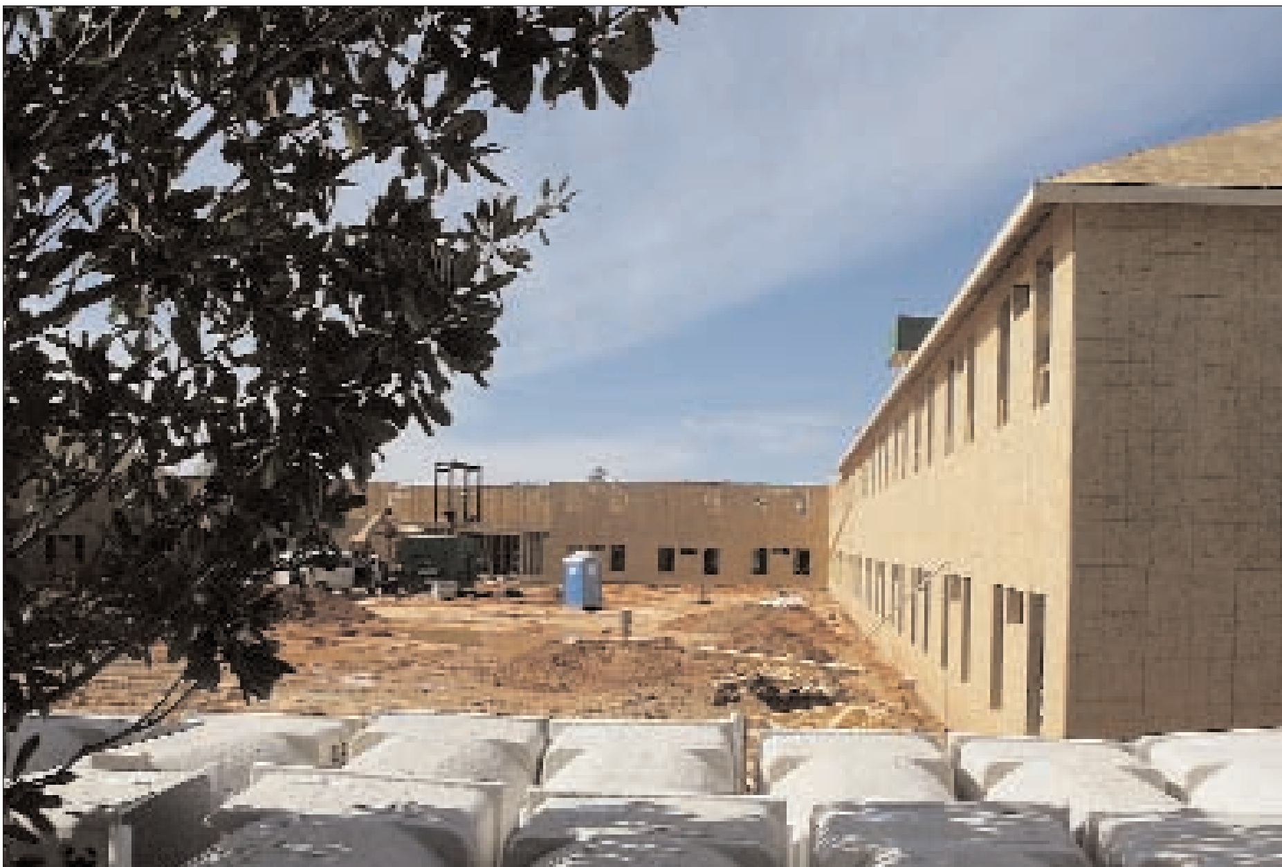
Construction on a new women's dormitory (168 rooms) and a men's dormitory (114 rooms) on the Poplarville campus began in July, 2005. They are expected to be complete by August, 2006. Each room will be semi-private with its own bathroom. The dormitories will have two stories. The dorms were designed by Hattiesburg architect Don McCleskey. The general contractor is Witherington Construction Co., of Mobile, Ala. Photos by Mitch Deaver
