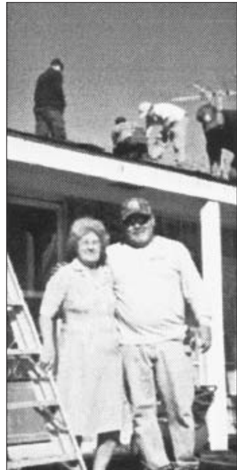
POPLARVILLE - Dale Miller, instructor of Automation and Controls at PRCC, poses with Mable Riles of Sones Chapel while PRCC students work to replace her torn roof. Miller said he believes anyone who gets involved in volunteer service will reap benefits far beyond graduation.
