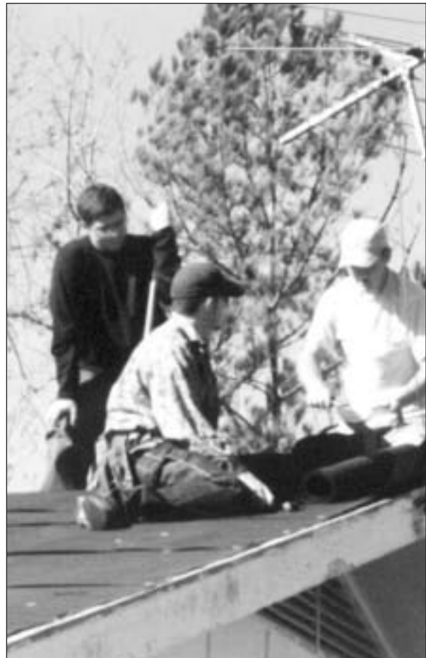
POPLARVILLE - From left, Anthony Vitale IV of McNeill, Eric Anderson of Mobile, Ala. and Dwight Lee of Leetown, PRCC students in the Automation and Controls program, work on 84-year-old Mable Riles' roof in Sones Chapel in January. PRCC students volunteered to help replace Riles's roof, which was damaged by Hurricane Katrina.
