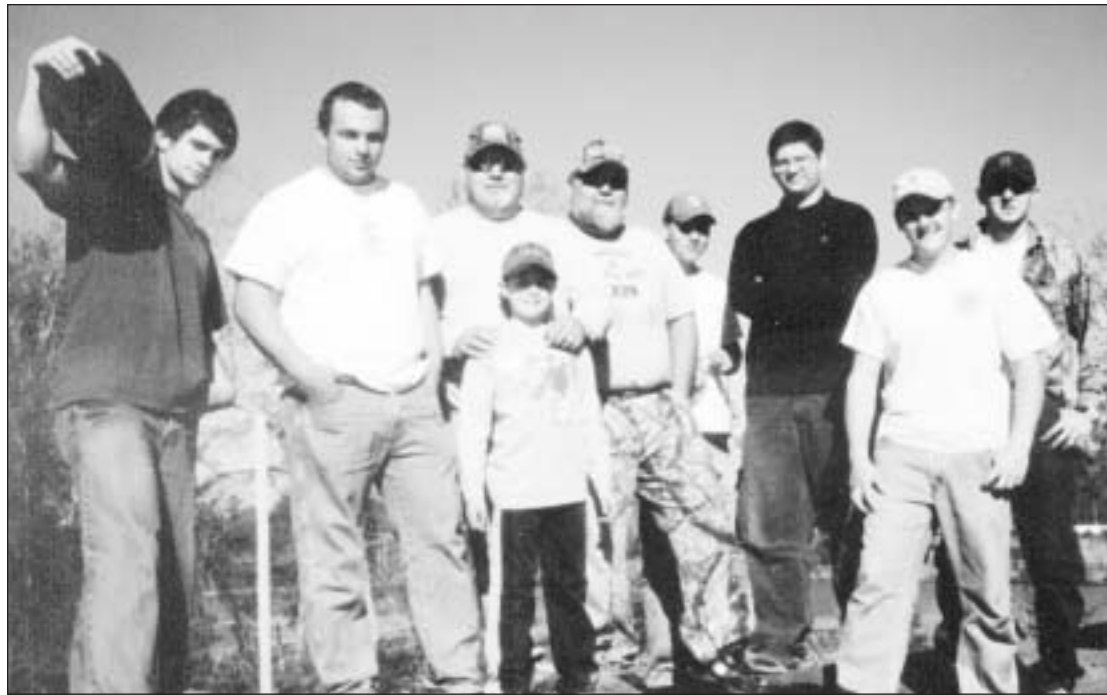
POPLARVILLE - Mable Riles of Sones Chapel in Pearl River County had a host of Pearl River Community College instructors and students on her roof recently. The group volunteered to replace the 84-year-old Riles' roof, which was damaged by Hurricane Katrina. The group included, from left, Jarred Bragg and Dwight Sick of Bay St. Louis, Dale Miller, instructor in the Automation and Controls program at PRCC, Miller's his 7-year-old son, Cody, Leland Kennedy, instructor in the welding department at PRCC, Justin Mooney of Carriere, Anthony Vitale IV of McNeill, Dwight Lee of Leetown and Eric Anderson of Mobile, Ala.
