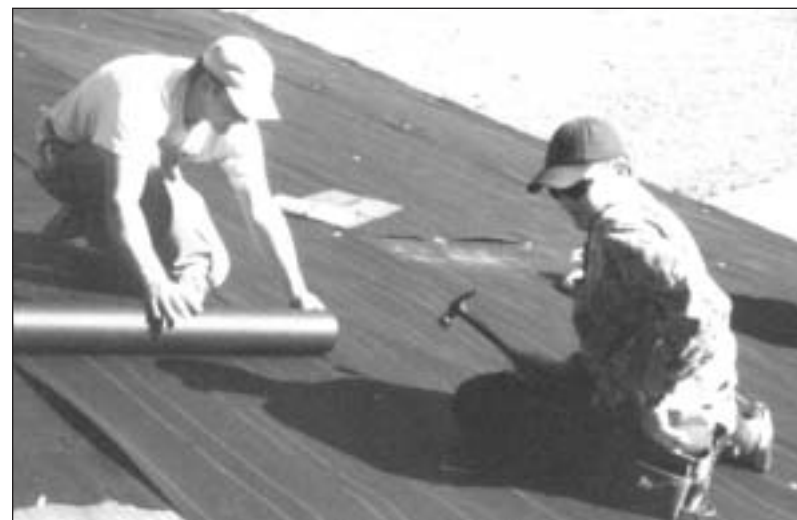
POPLARVILLE - Dwight Lee (left) of Leetown and Eric Anderson of Mobile, Ala., PRCC students in the Automation and Controls program, work on 84-year-old Mable Riles' roof in Sones Chapel in January. Lee, Anderson and other PRCC students volunteered to help replace Riles's roof, which was damaged by Hurricane Katrina.
