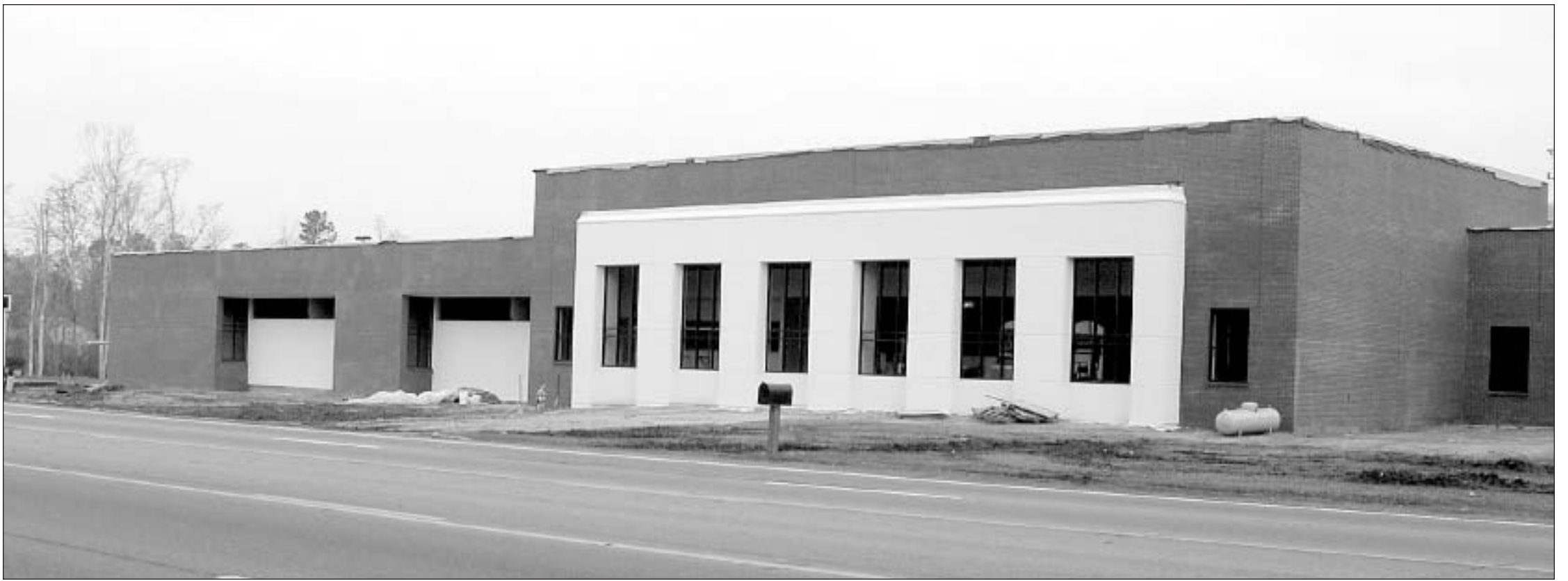
Despite Hurricane Katrina's interruption, construction continues on the new building at the Forrest County Center in Hattiesburg. The 12,000 square-foot building across the front of the campus on U.S. 49 South will provide a new academic image to the school. New spaces include five classrooms, a learning center with 30-35 computers, new library space with two study rooms and administrative space, two new academic offices and new restrooms. The photograph above is from the back of the building. Completion of the project is expected to be sometime in late spring, 2006.
