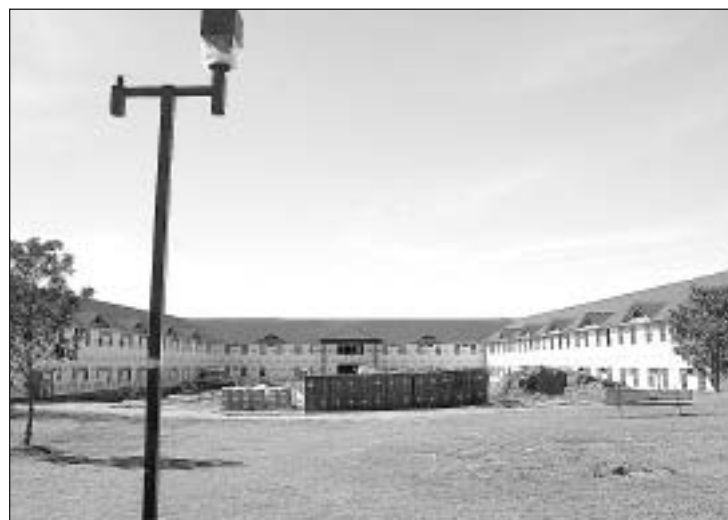
GETTING READY: Construction work on two new dormitories on the Poplarville campus and a classroom-library building at the Forrest County Center in Hattiesburg that began before Katrina is going strong today.
