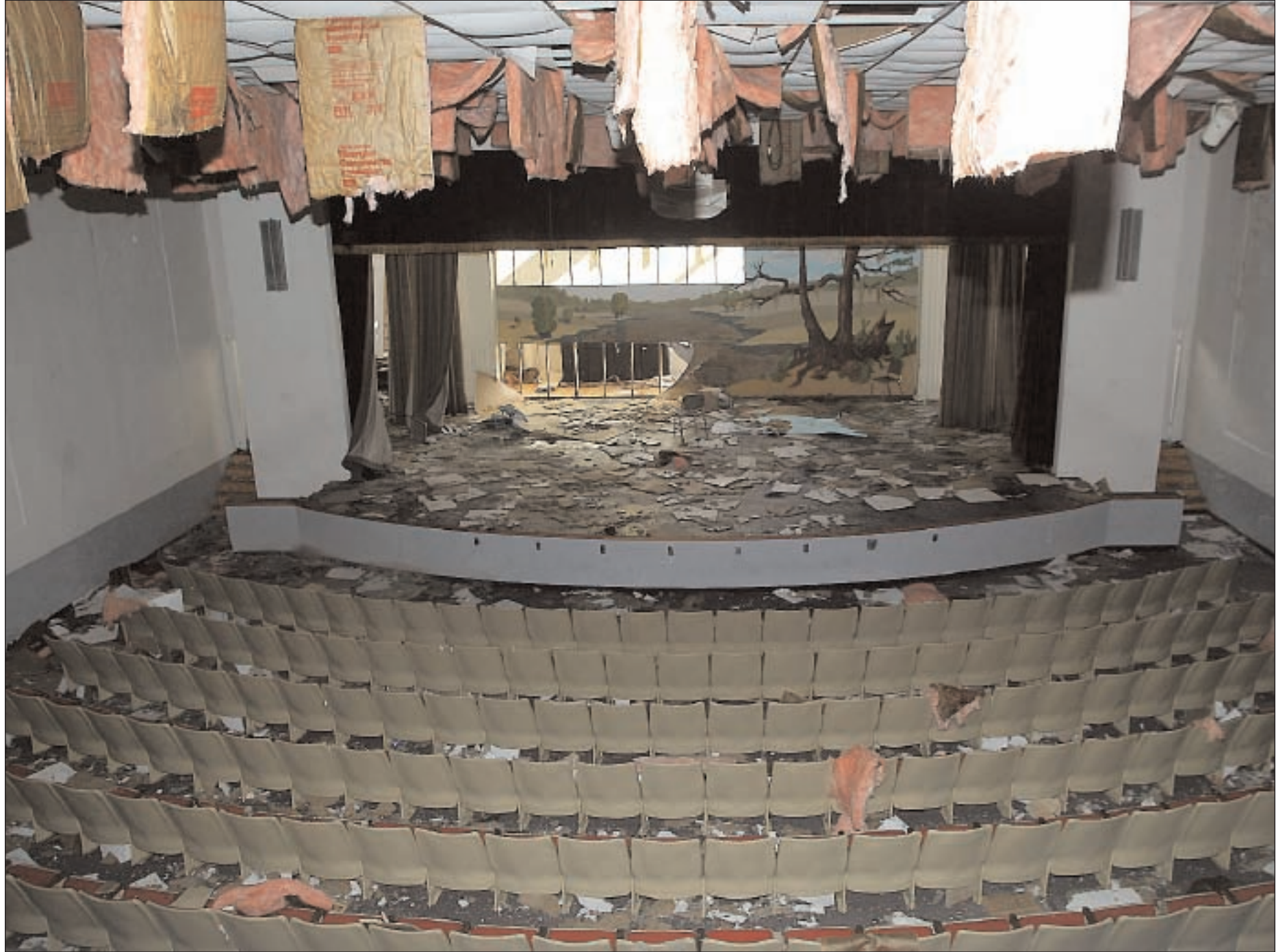
POPLARVILLE - Moody Hall, a three-story structure built in 1926 and the oldest classroom building among the state's 15 community and junior colleges, suffered heavy damage from Katrina. The auditorium roof blew off during the height of the storm, resulting in extensive interior damage from wind and rain. Photo by Mitch Deaver.
