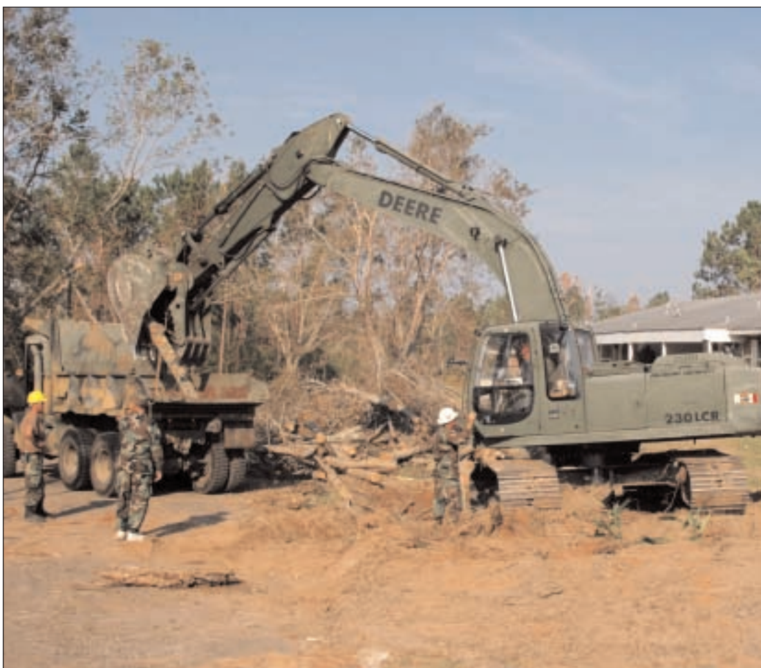
Pictured working on Faculty Row, the 890th Engineer Battalion, with men from Picayune, Columbia, Purvis, Lumberton, and Hancock County, removed debris from throughout the campus.
