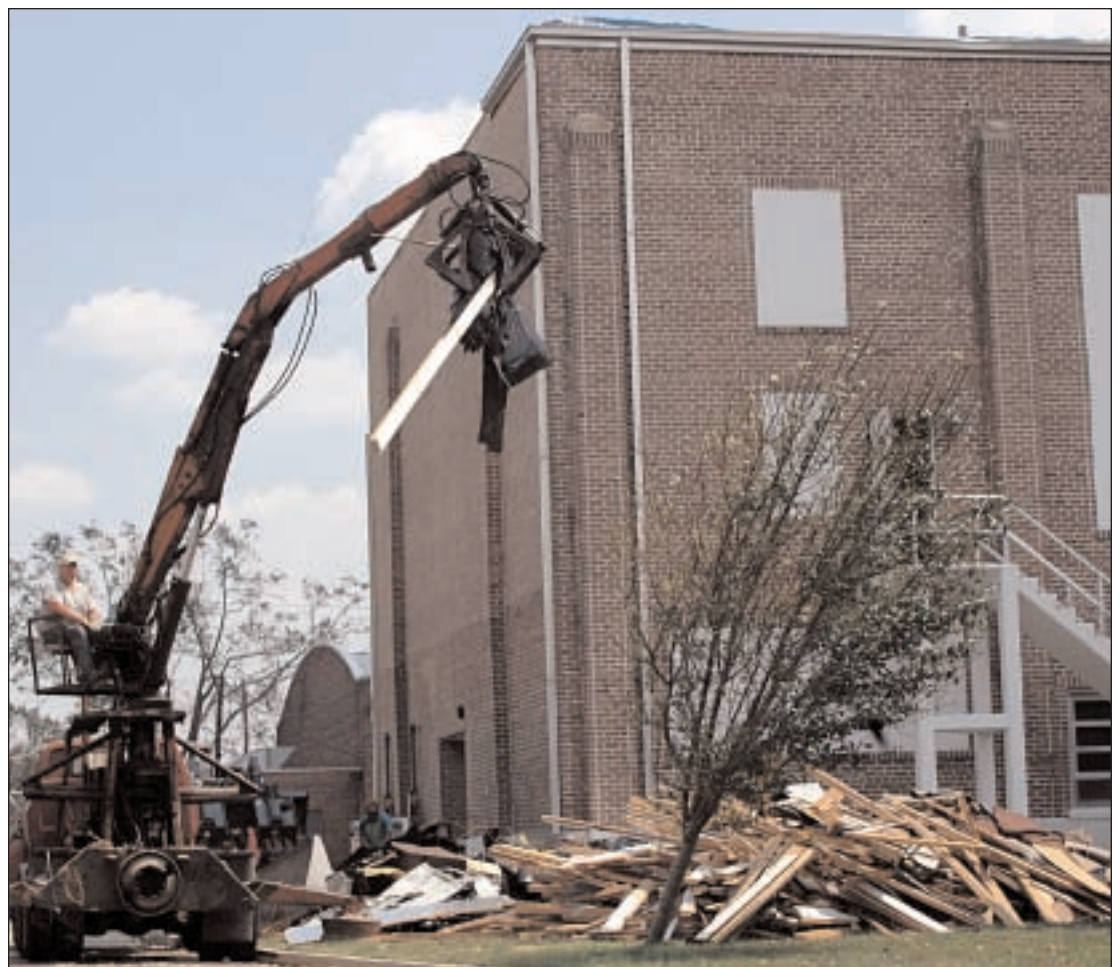
Contractors had a huge pile of debris to remove from Moody Hall. Most of the debris was the roof that was once over the stage and ceilings from faculty offices located on the first floor.
