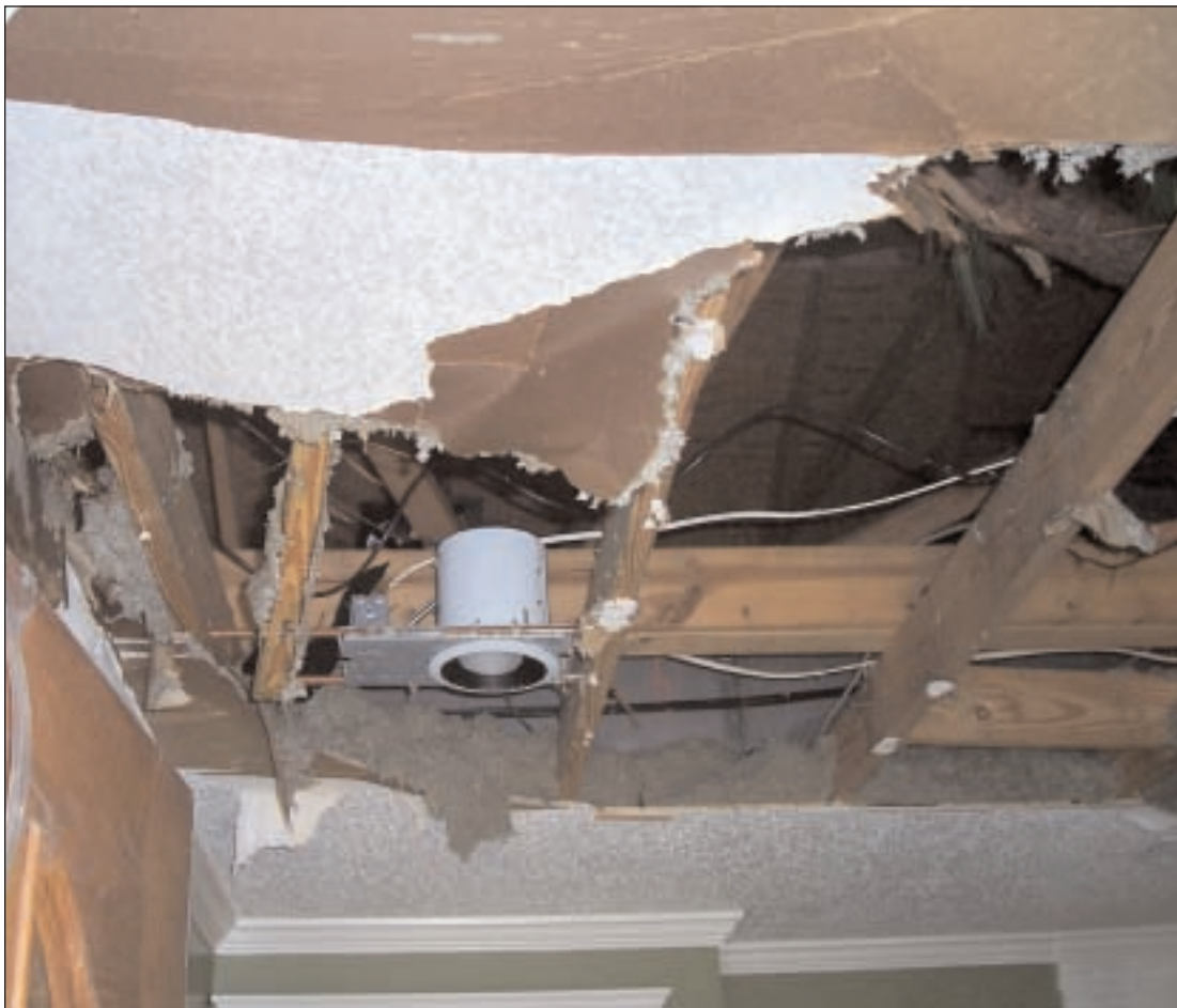
Academic Counselor Ethel Batson's home in Poplarville suffered extensive interior damage.
