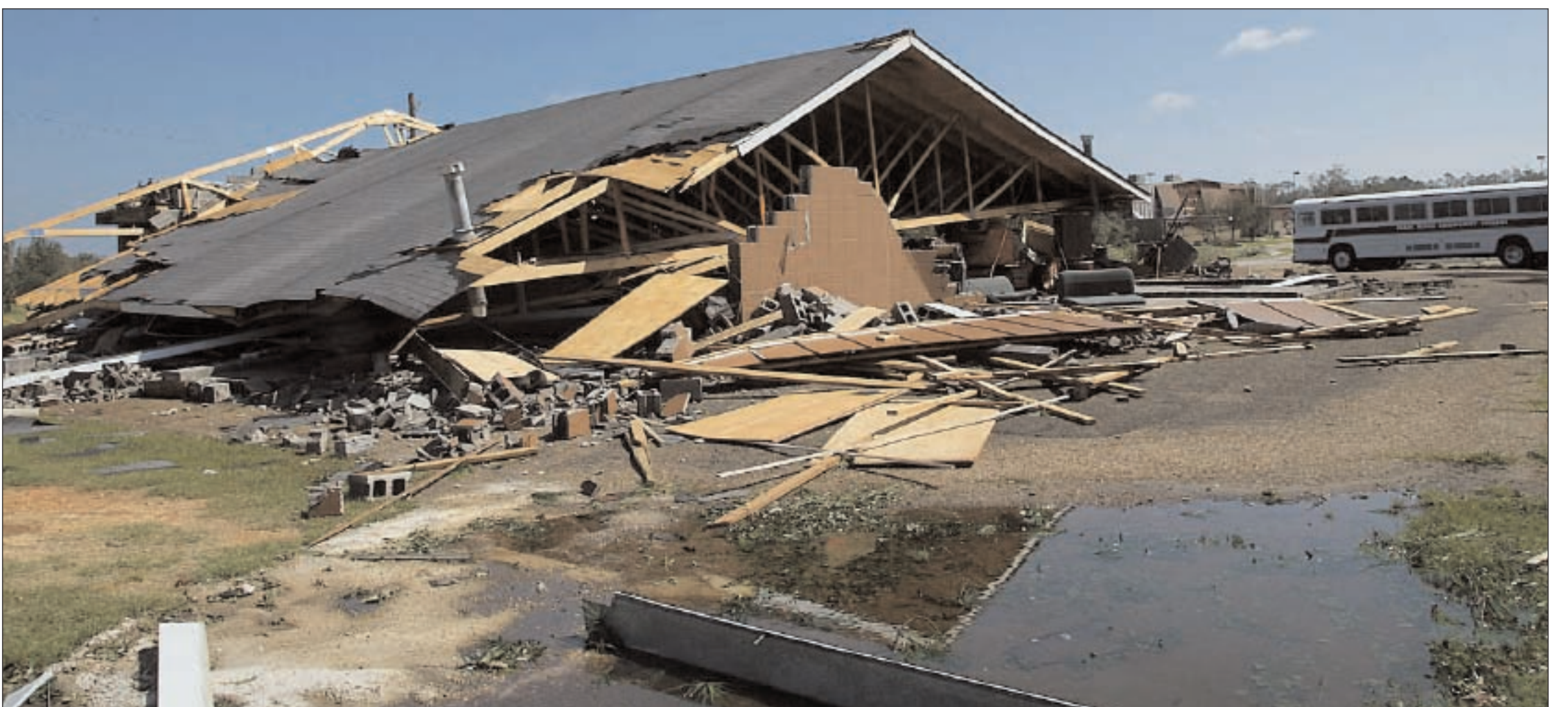
POPLARVILLE - The PRCC bus barn was completely destroyed by winds that reached 120 miles-per-hour on campus.
