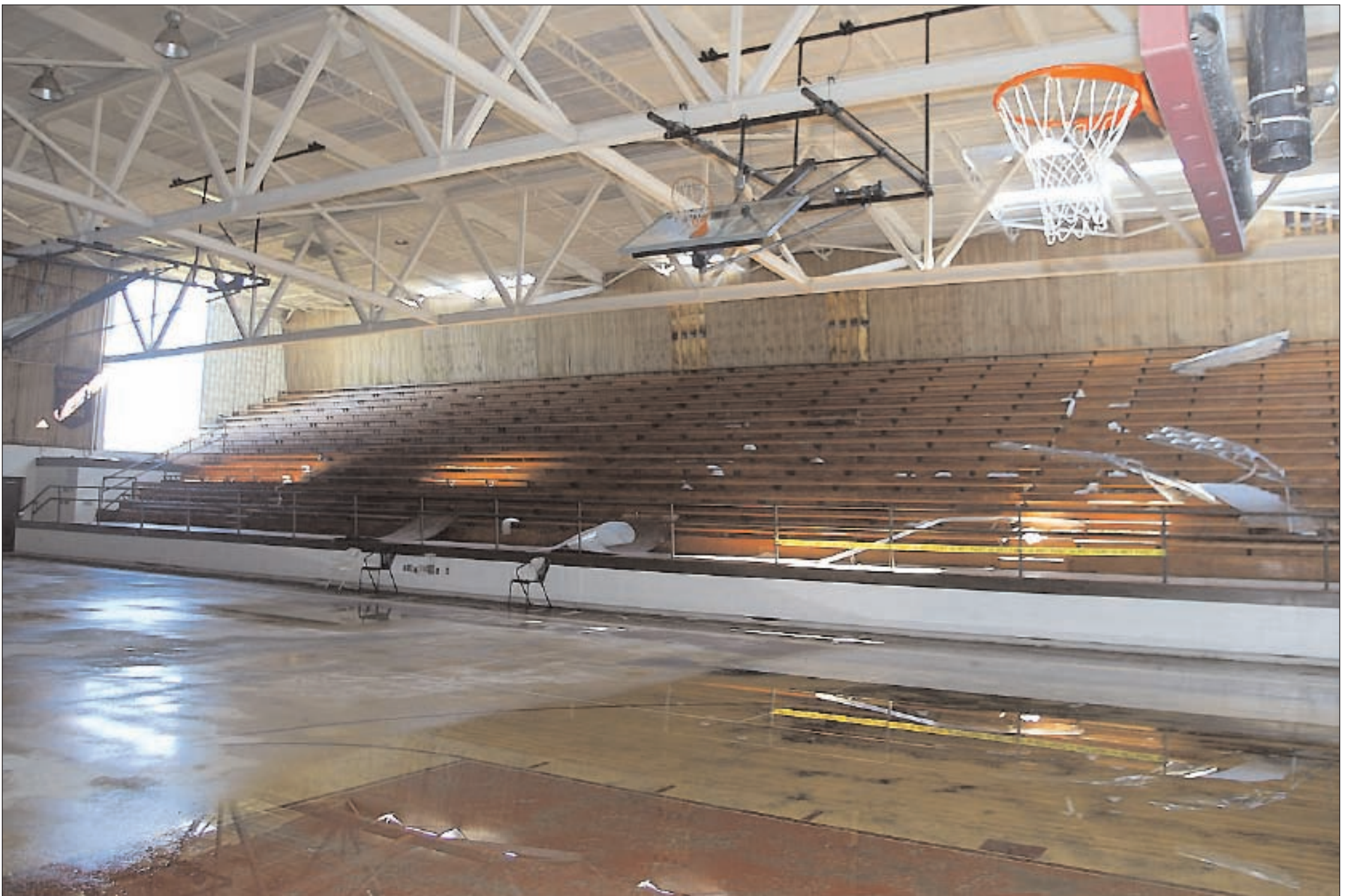
POPLARVILLE - The 2005-06 Wildcat basketball teams will have to find a new home for the rest of this school year and possibly the next. M.R. White Coliseum, which was built in 1974, suffered extensive interior and exterior damage. The early recommendation is that White Coliseum, home to such events as graduation and the annual Extravaganza, will have to be torn down.
