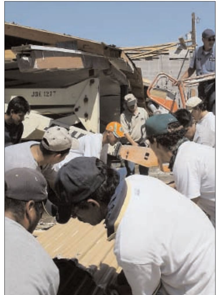
Workers take down what's left of the Vehicle Maintenance Shop, which was demolished by Hurricane Katrina.
