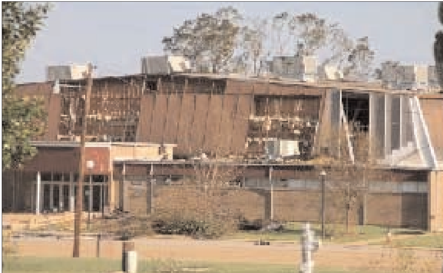
Daylight the morning after Hurricane Katrina revealed just how much damage was done to M.R. White Coliseum, home of graduation each year.
